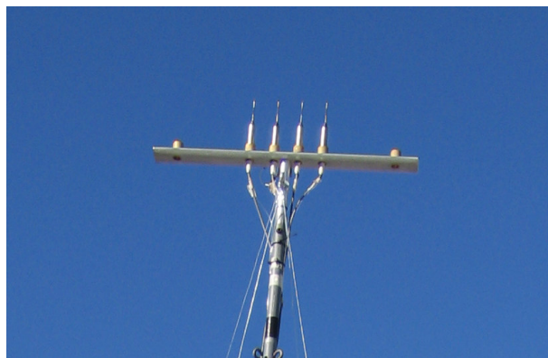
Figure 32: Probe bracket fitted to mast with probes in situ.
